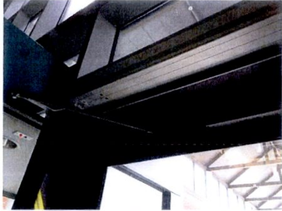
Close up view of the electronic assist exit device. Push button devices and power will be installed after doors and hardware are complete.
