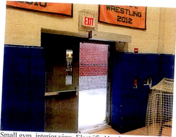
Small gym, interior view. Electrified hardware is installed and needs to be wired.
