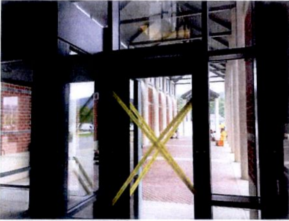
Rear Entrance of NMHS facing east (towards Athletic Fields). Note the new door and electronic assist device mounted to the frame. Push button devices and power will be installed after doors and hardware are complete.
