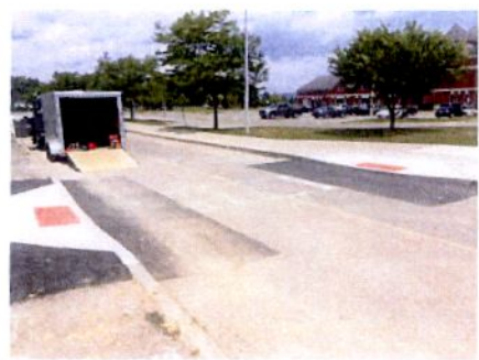
New drop curbs to access both the new turf fields and NMHS on either side of the roadway.
