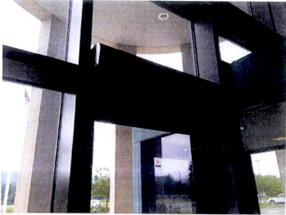
Main entrance to NMHS facing east. New door and actuator. Push button devices and power will be installed after doors and hardware are complete.
