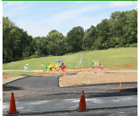
Final preparations are being made to the restructured parking lot/playground area at Hill and Plain school.
