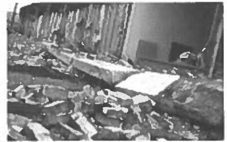
Earthquake damage in Washington in 2001
